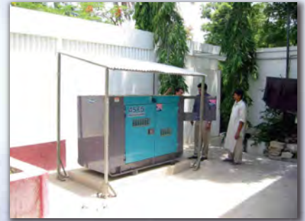
As the Emergency power source in the hospital.
