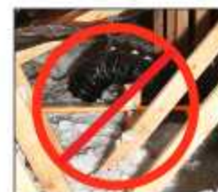
INCORRECT (Exposed piping)
