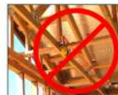
INCORRECT (Unconditioned at rough-in)
